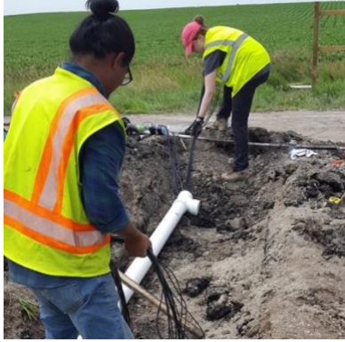
Figure 3.13 Pulling the cables through fittings and PVC pipes at the bottom of the trench in subgrade.
