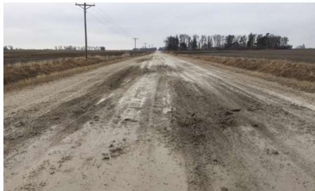
Figure 1.1 Damaged granular-surfaced roadway due to freeze-thaw cycles in Hamilton County, Iowa.
