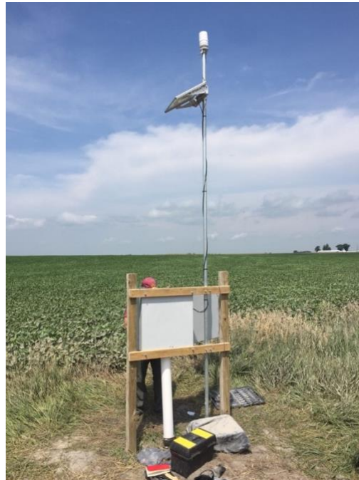
Figure 3.3 Installation of the weather station at the top of the steel tube.
