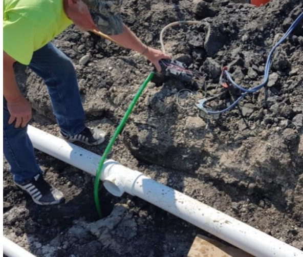
Figure 3.15 12-Volt water pump used to discharge groundwater.
