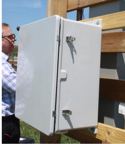
Figure 3.1 Enclosure used in Hamilton site to protect DAQ equipment.
