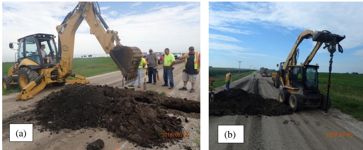
Figure 3.8 Heavy construction equipment used in Hamilton site installation: (a) backhoe for trenching, (b) skid-steer for the borehole drilling.
