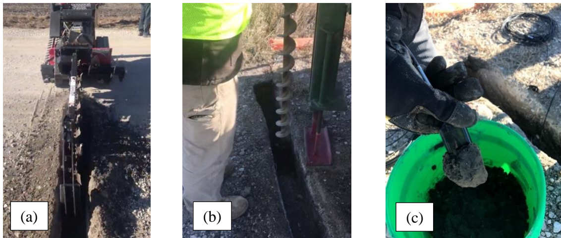
Figure 4.2 Installation of replacement sensors in January 2019: (a) digging the trench with a trencher, (b) drilling the boreholes, (c) packing MPS6 sensors with native soil.
